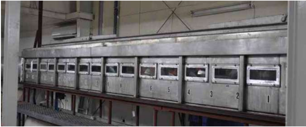
STEINER TUNNEL FIRE MACHINE
