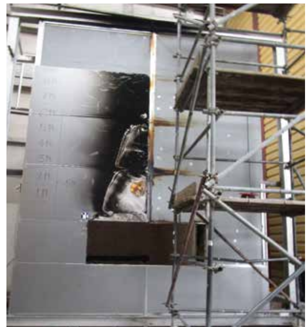
WALL CAVITY IN WALL ASSEMBLY AFTER FIRE TEST
